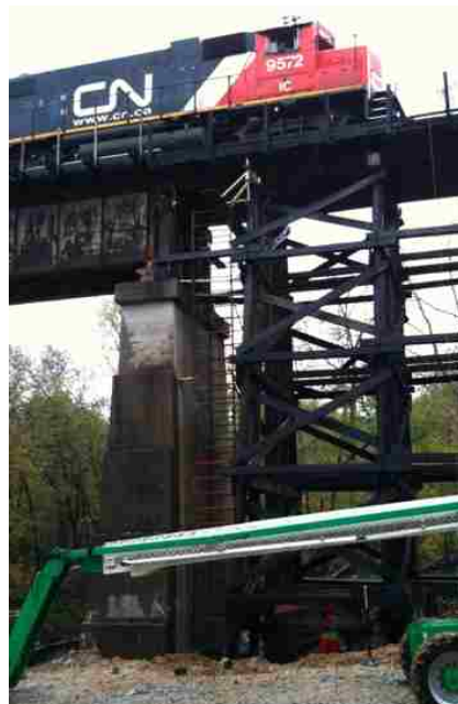
Fig. 2.2. Scaffolding to provide fixed reference point for displacement measurement of a railroad bridge (Moreu et al. 2015).
